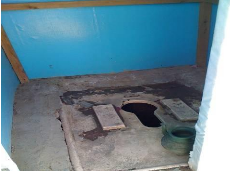
VIP latrine in new durrani camp
